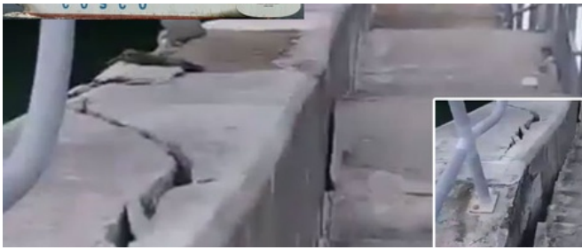
Neopanamax container ship collided with Panama Canal Lock wall
